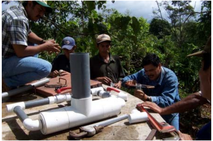
Field installation of a CTI 8 chlorinator.
