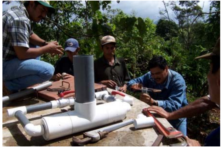
Field installation of a CTI 8 chlorinator.
