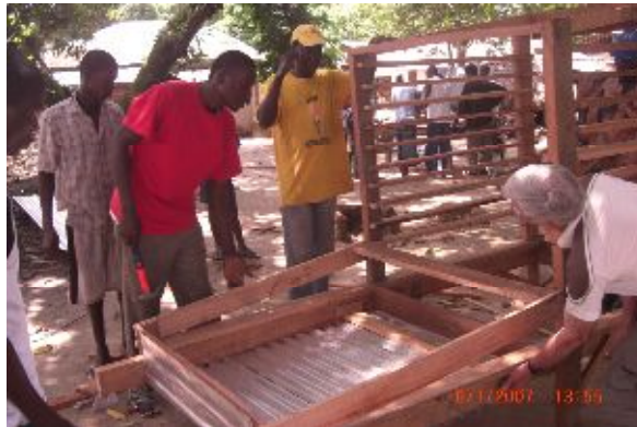
The framework and back view of the solar dryer. Ed Galle (far right) instructs Fallah Saah (red shirt) and Barwain Zayzay (yellow shirt) on construction techniques
